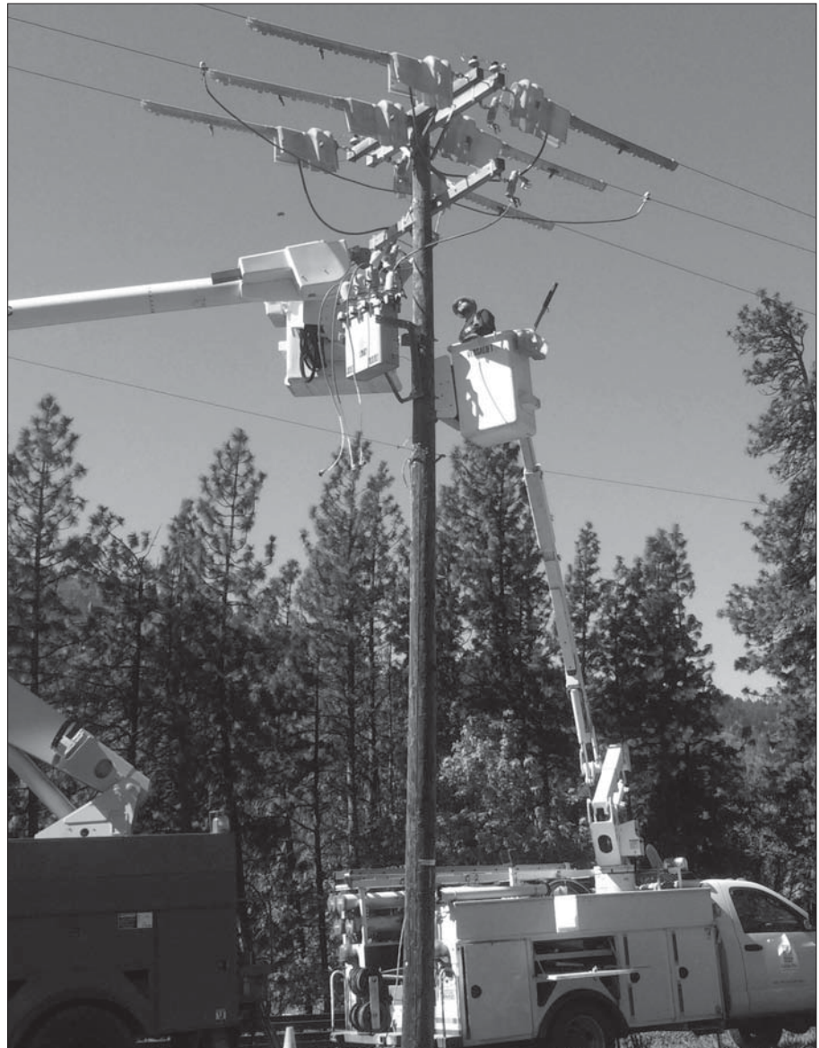
Klickitat PUD linemen Justen Greenwood and TJ Lutz work on a new location for the Burdoin breaker. The line is energized and they are using live line tools to install the device without interrupting service.
